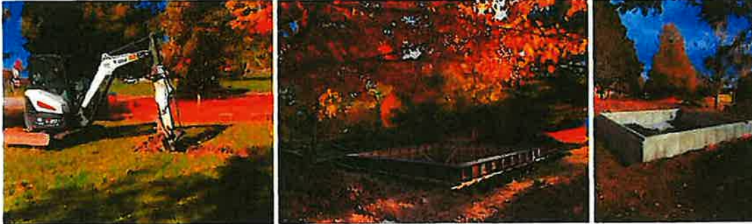
From left to right: ground breaking scoop on November 2, preliminary foundation completed on November 4, and current finished foundation.
